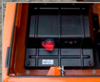
Battery cut-off switch
